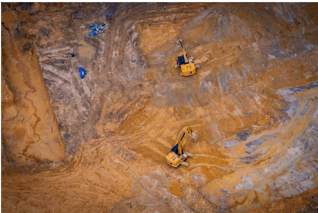
PHOTO 5 – BACKHOES IN OPERATION AT YANOMAMI INDIGENOUS TERRITORY, ON DECEMBER 2022. CREDIT: VALENTINA RICARDO (HAY/GREENPEACE)
