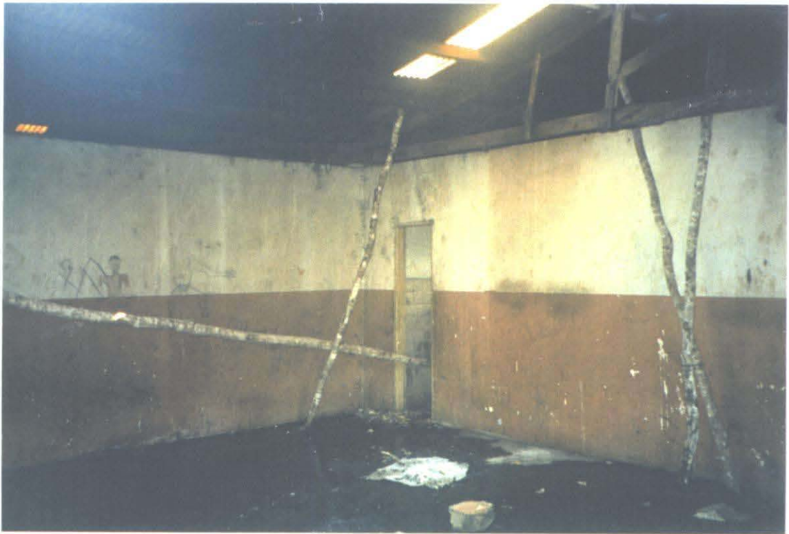
8. Posto Leonardo in disrepair
